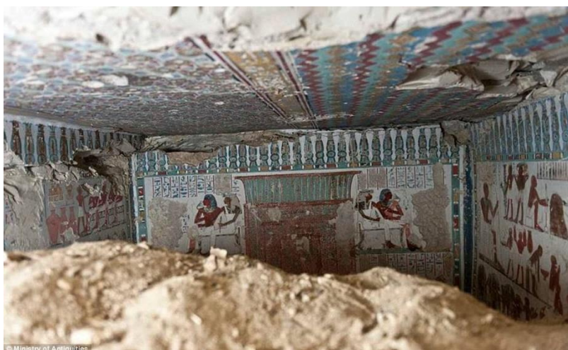
Figure 21.18 Tomb with collapsed ceiling and cracks in walls
